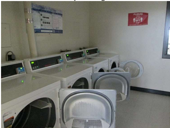
Subject central laundry facility
