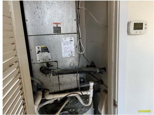
Existing In-Unit Mechanicals
