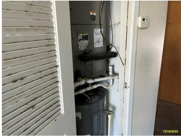
Existing In-Unit Mechanicals
